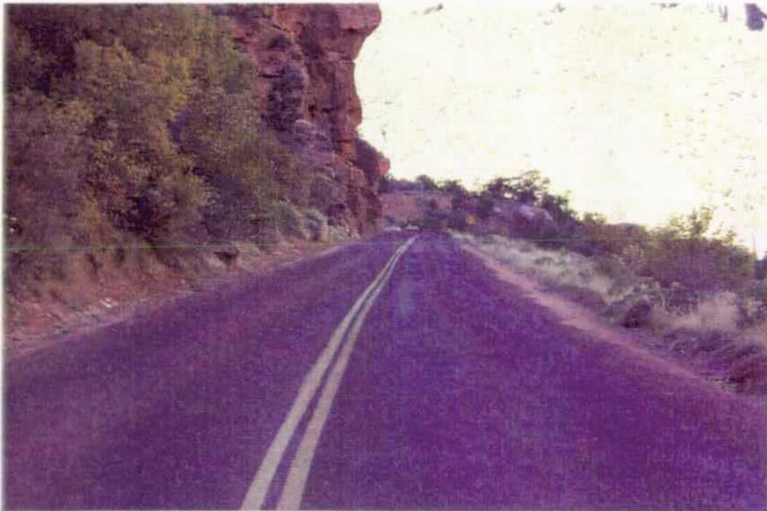
Photo #17 - MP 2.10 - Longitudinal Cracks, sealed transverse cracks..
