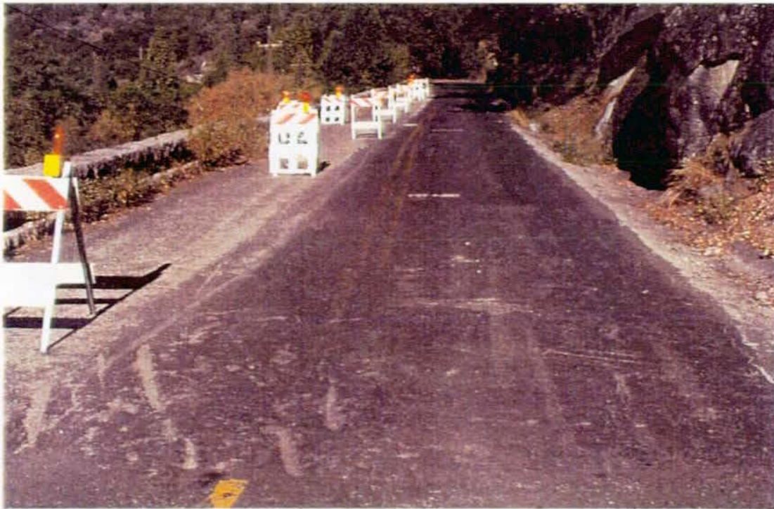
Photo #3457 - MP 5.60 - Shoulder Washout
