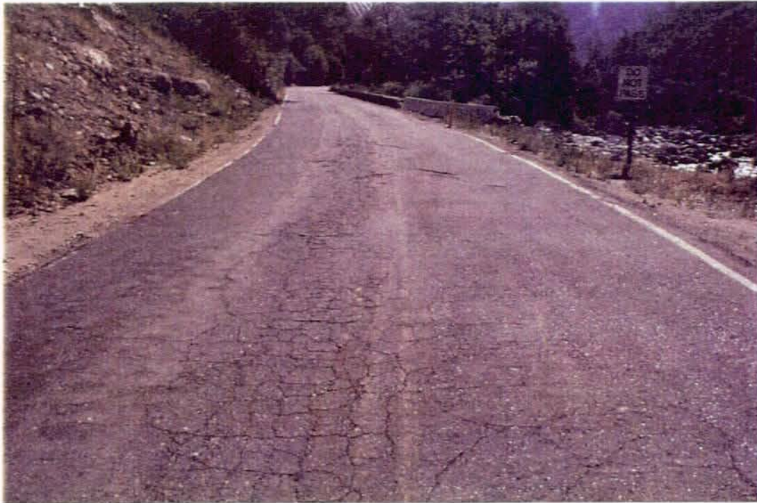
Photo #3439 - MP 0.00 - Begin at Park Boundary. Note alligator cracking.
