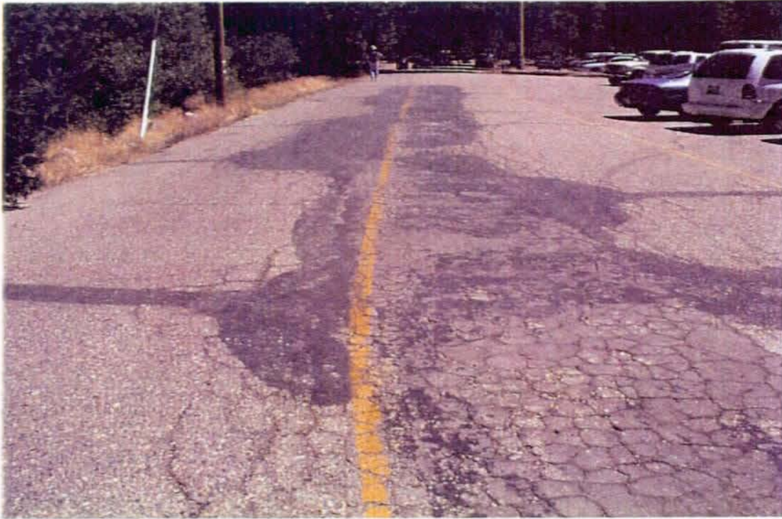
Photo #3442 - MP 0.00 - Begin at Rte 014. Heavy alligator cracking.
