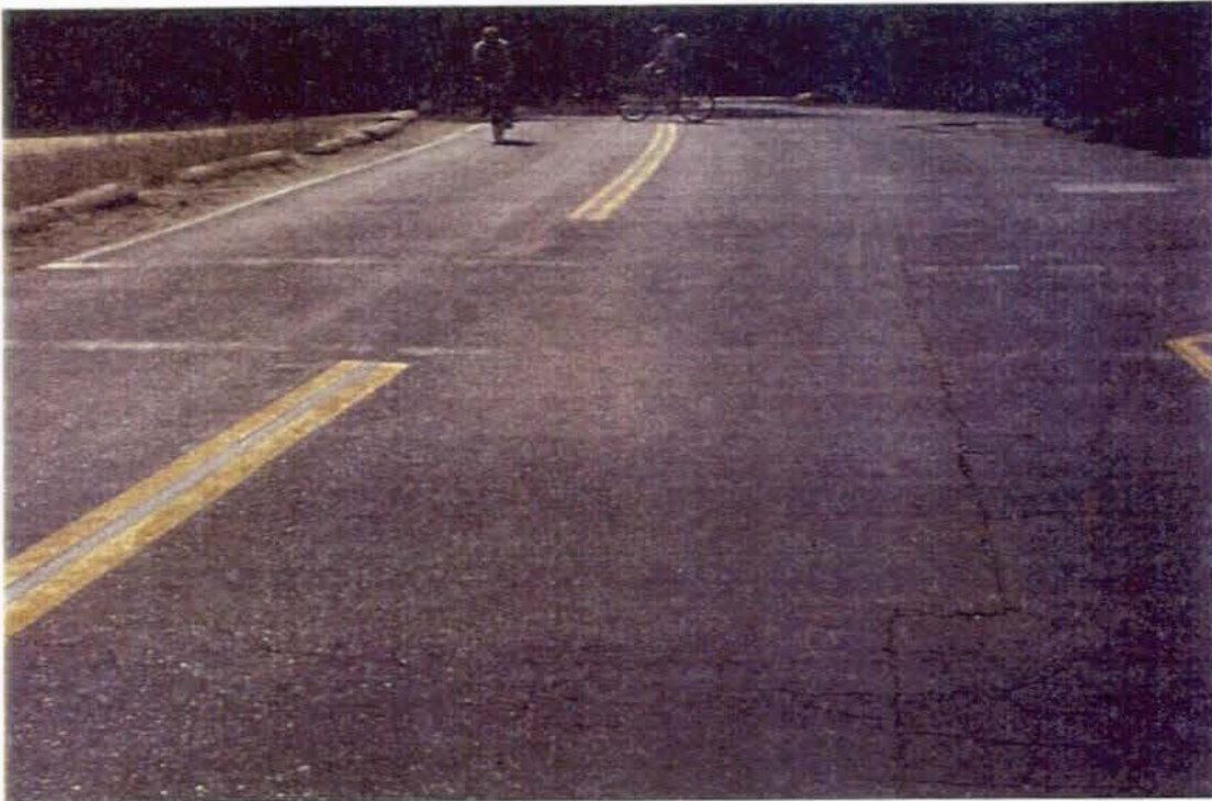
Photo #3463 - MP 0.00 - Begin at Rte 500. Note right side block cracking.
