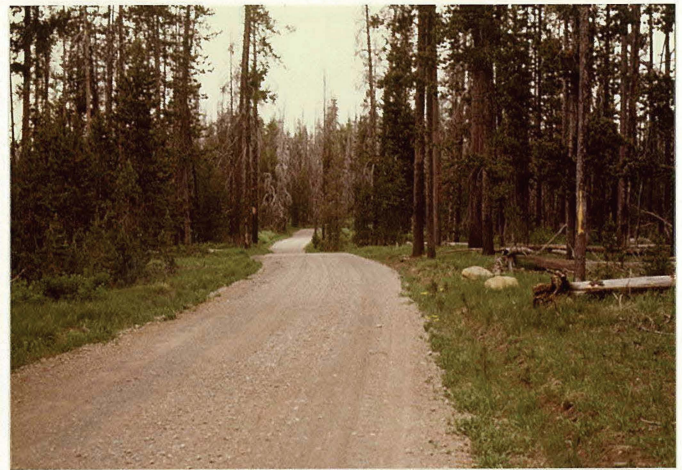
MP 0.44 Typical Roadway Condition
