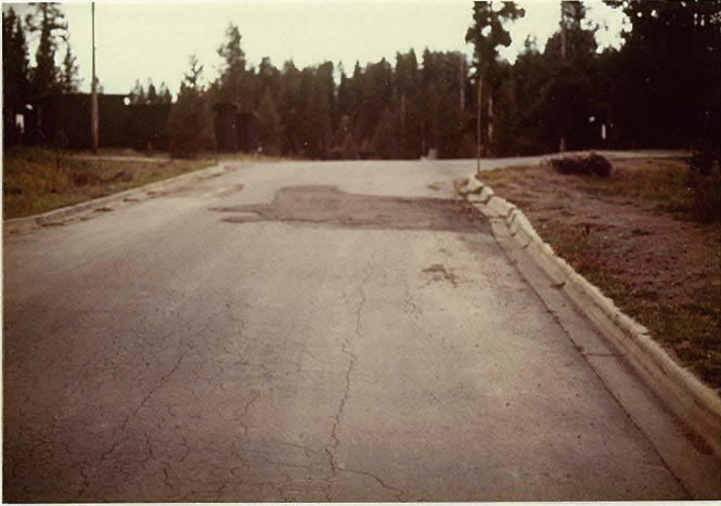
MP 0.37 Base Failure Under Roadway and Curb
