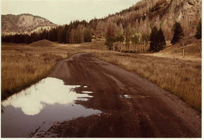
MP 0.91 Poor Roadway Drainage
