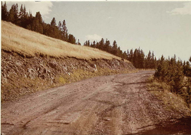
MP 0.71 Typical Rough and Rutted Roadway
