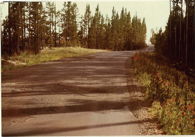
MP 1.01 Roadway Base Failure
