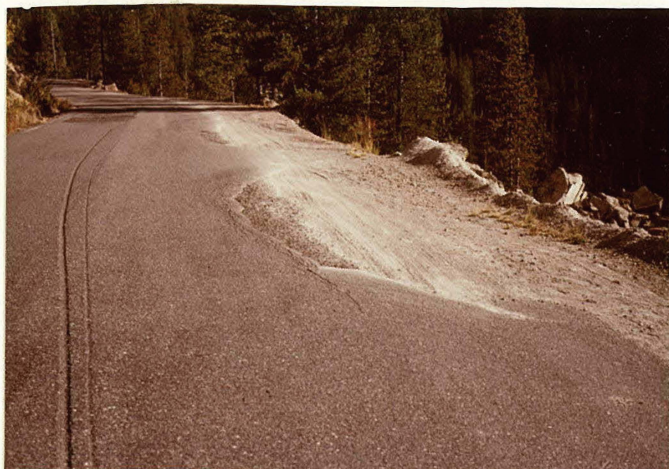
MP 0.86 Road Failure Above Timber Cribwall
