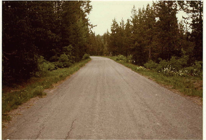
MP 0.12 Typical Roadway Condition
