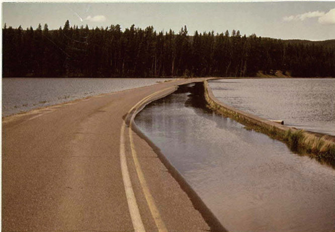
MP 0.55 Facing Northwest, Roadway Flooded by Yellowstone Lake
