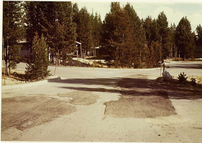
Roadway Failure in Cabins Area
