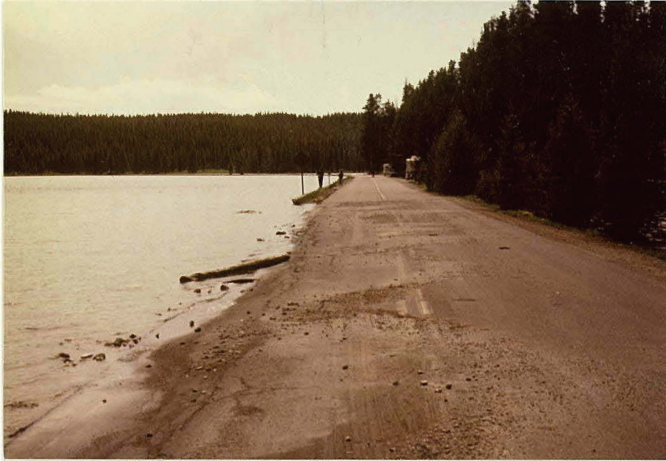
MP 0.13 Roadway Flooded by Yellowstone Lake (June 1986)
