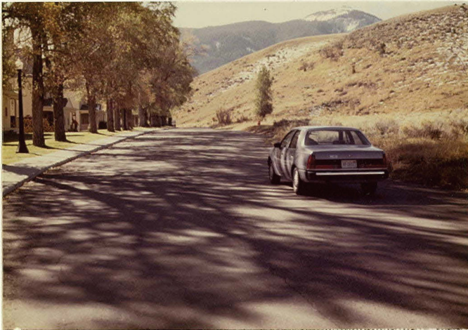
MP 0.09 Typical Road Condition at Park Headquarters
