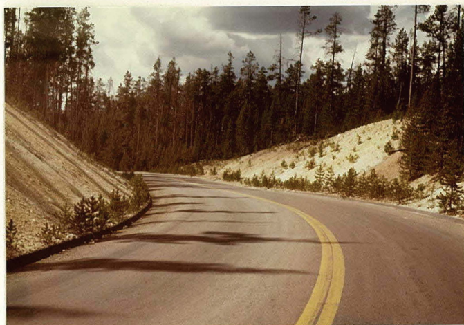
MP 1.18 Raveling Roadway Cut Slopes
