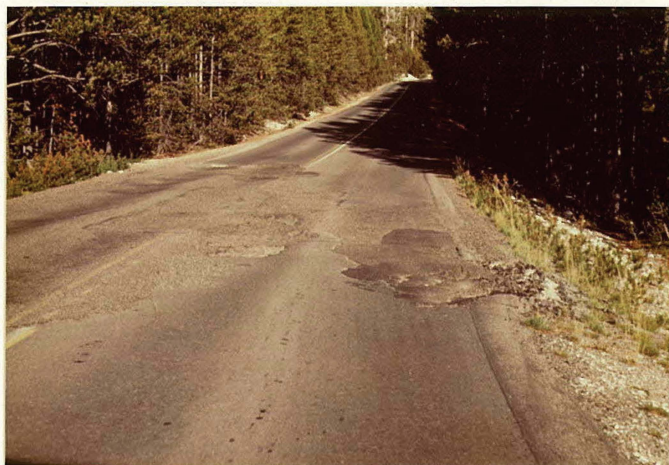
MP 0.26 Roadway Failure
