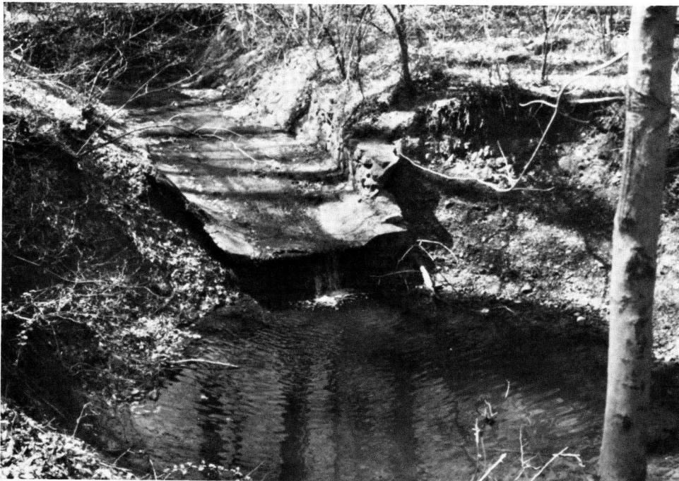
Figure 7-12 Scour at End of Concrete Apron
