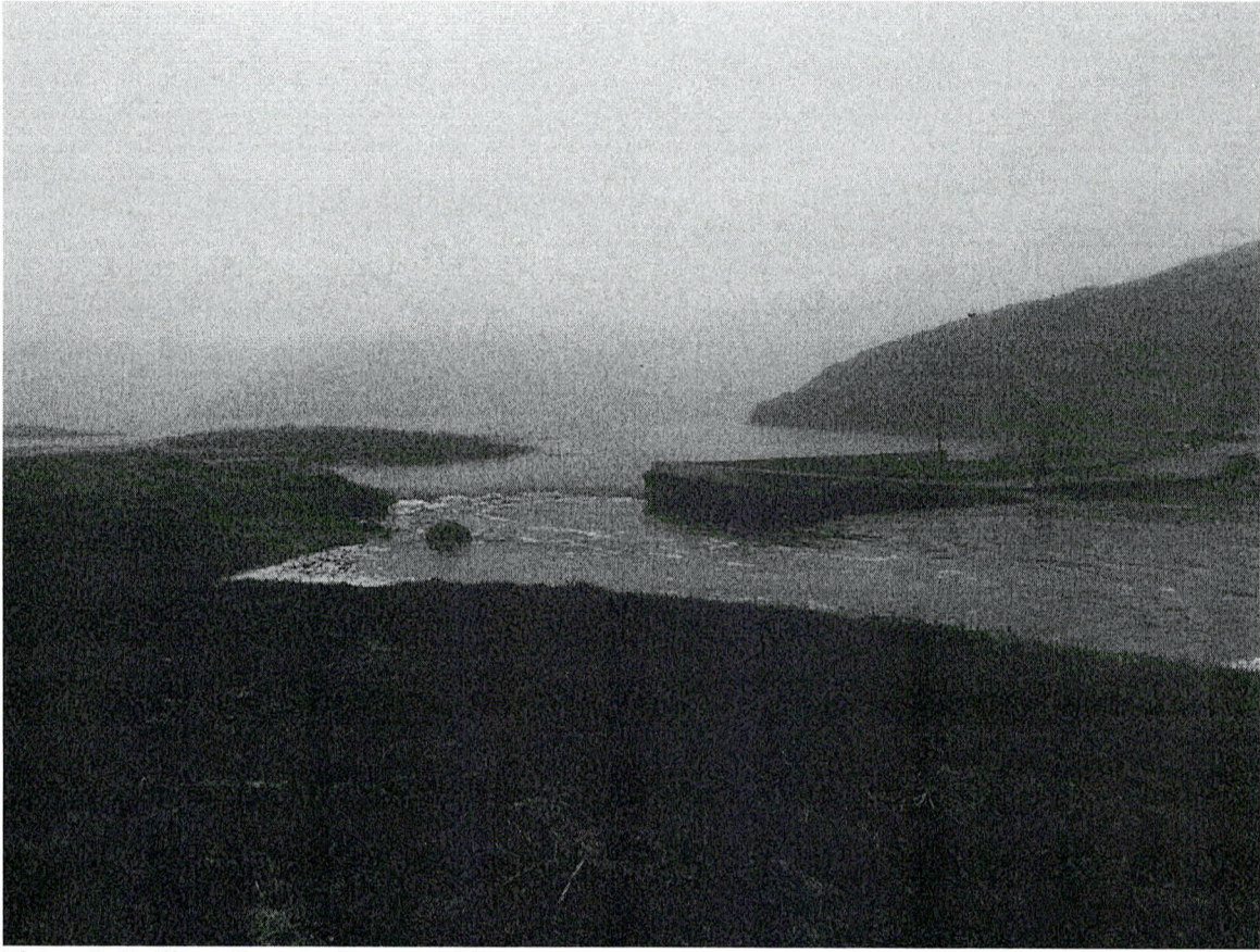
Figure 6. Spillway Breach - January 2002.
