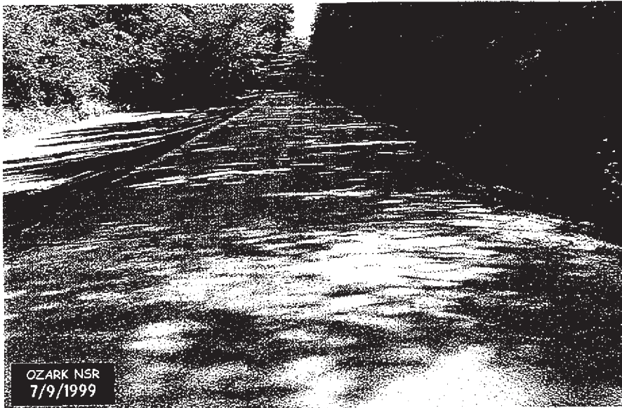
Photo # 15 – Route 125, Pavement Section Showing Utility Patch.
