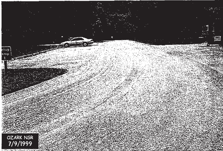
Photo # 19 – Route 217, Longitudinal Wheel Path Cracking.
