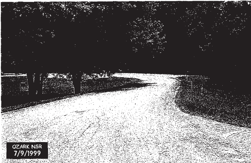
Photo # 18 – Longitudinal Cracks at Intersection.
