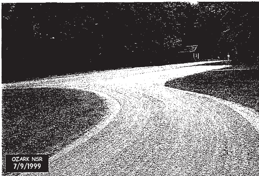
Photo # 20 – Route 217, Longitudinal Wheel Path Cracking.
