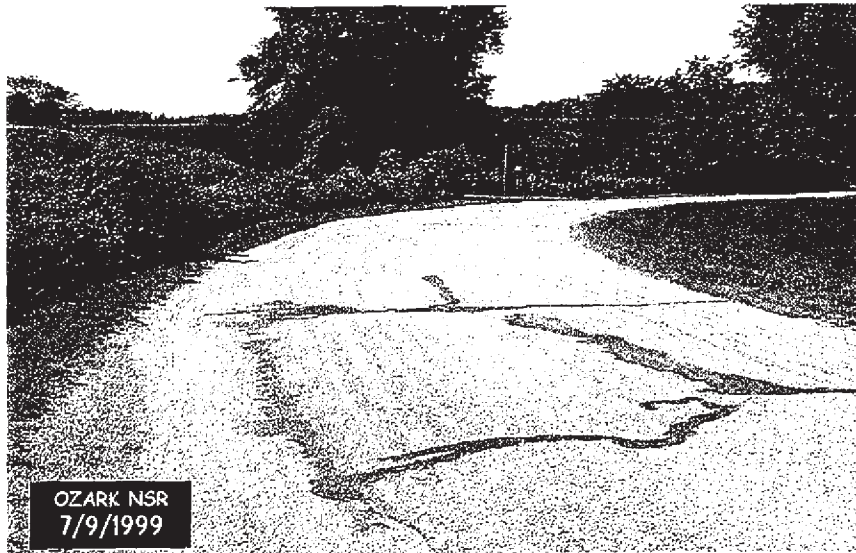
Photo # 23 -- Route 228, Sealed Cracks.
