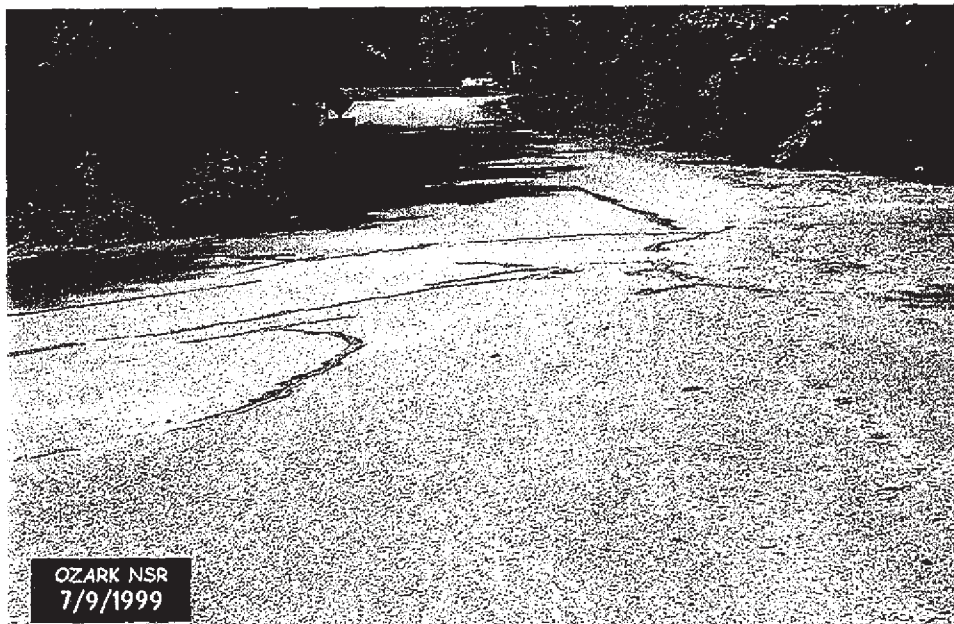
Photo # 06 -- Route 110, Typical Pavement Section Showing Sealed Cracks.
