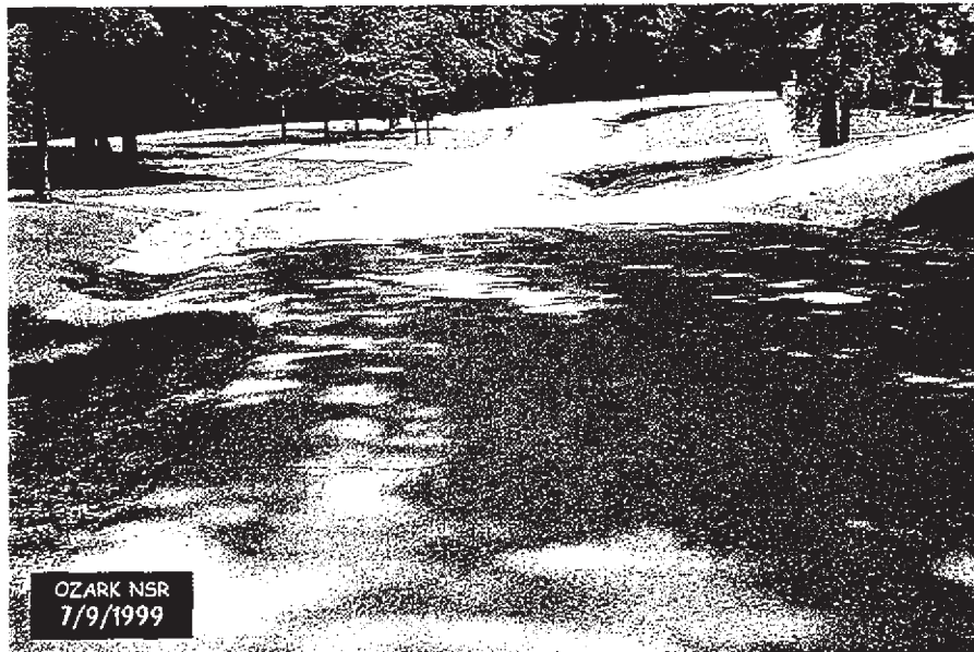
Photo # 28 – Route 417, Longitudinal and Transverse Cracking.
