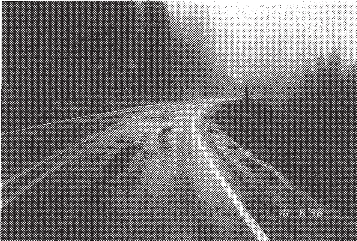
Photo R2-21 - MP 0.10 - Typical poor pavement
