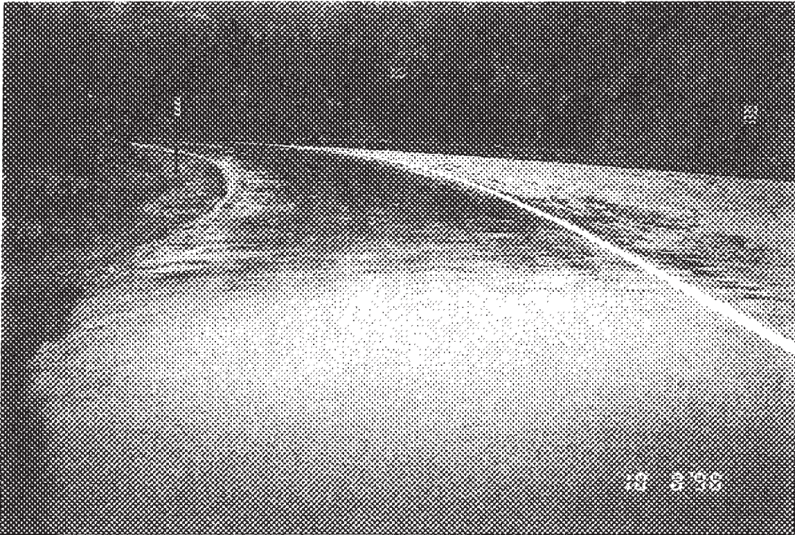
Photo R1-11 - MP 0.00 - Beginning of Rte at Rte 916/014, typical pavement section and rock wall
