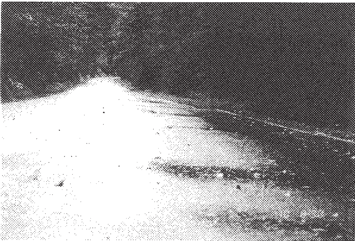
Photo R3-09 - MP 2.00 - Subgrade failure
