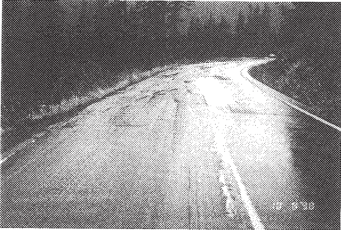
Photo R1-14 - MP 0.30 - Pavement distress slumping
