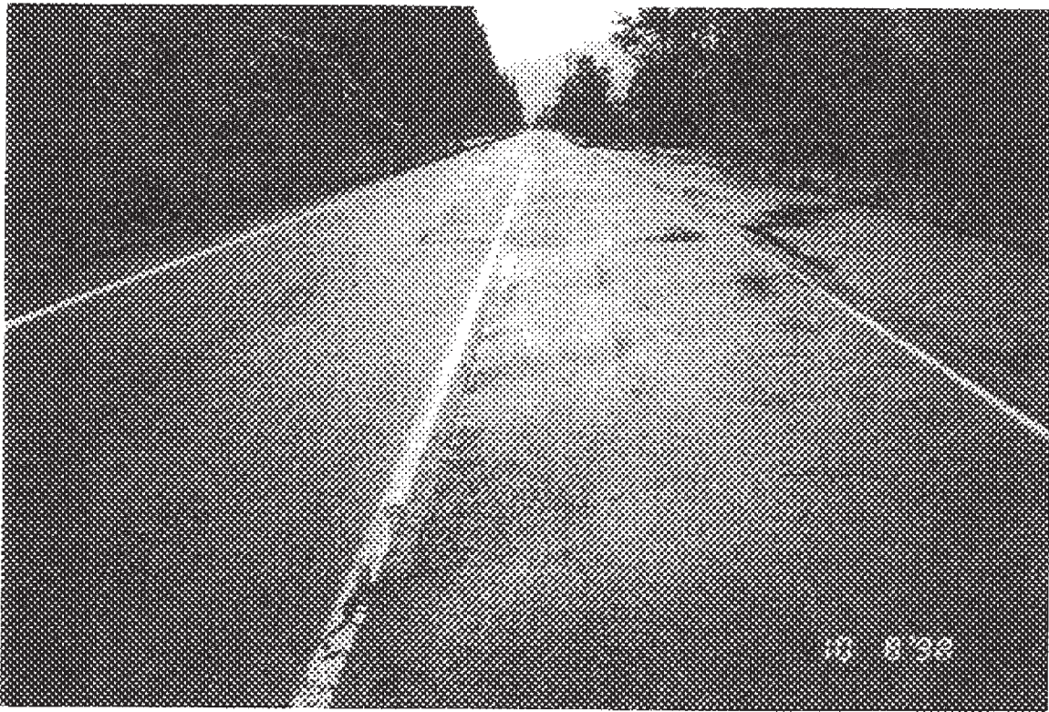
Photo R1-17 - MP 5.10 - Load related cracks in pavement
