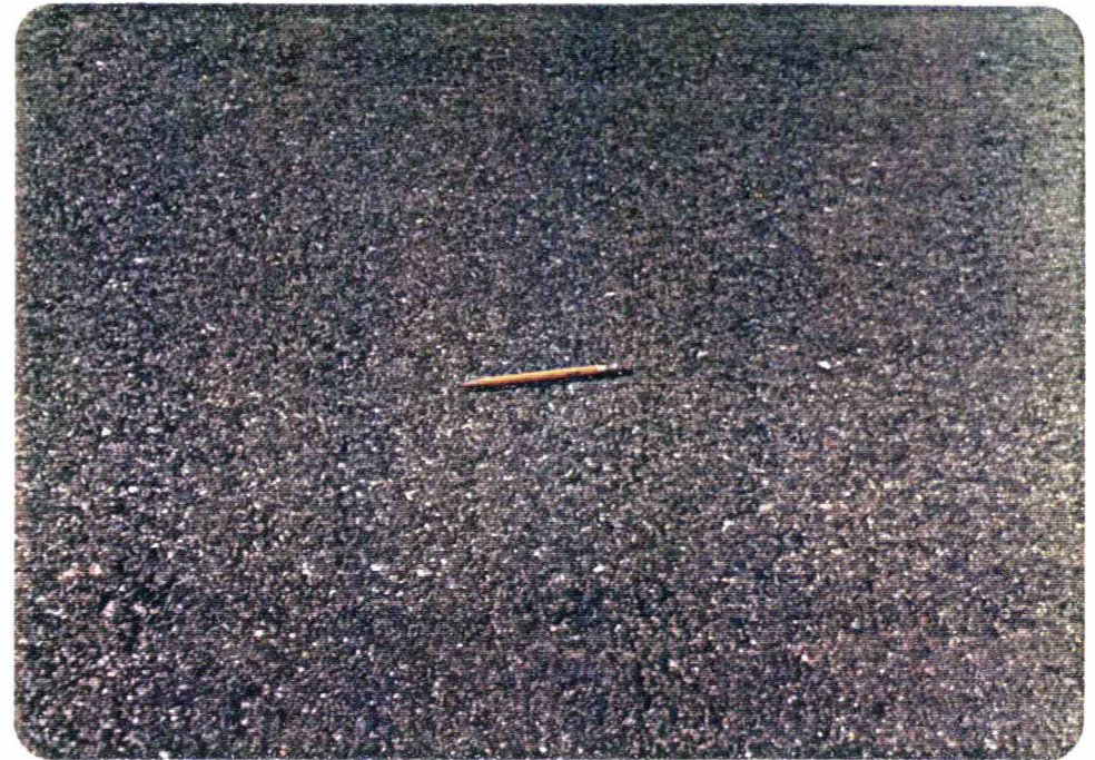
Raveling on Rte. 13
