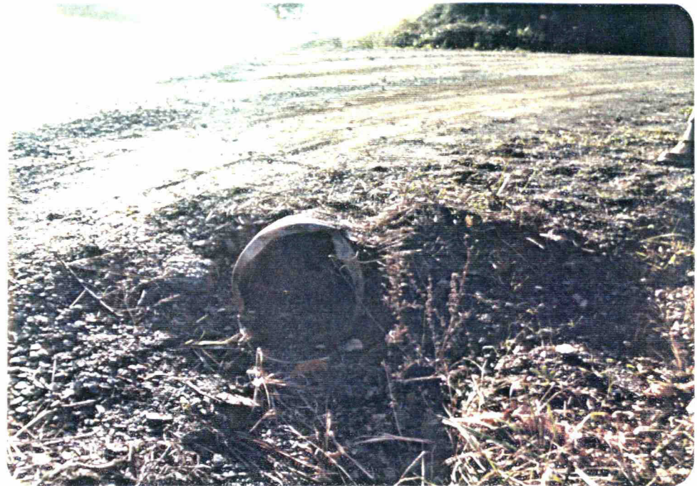
No Delineation of Culvert at Rte. 407 Intersection with U.S. 29
