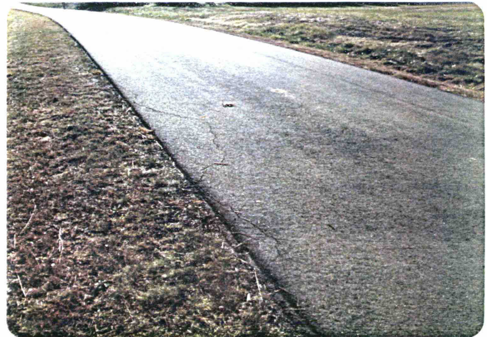
Edge Cracking along Rte 12
