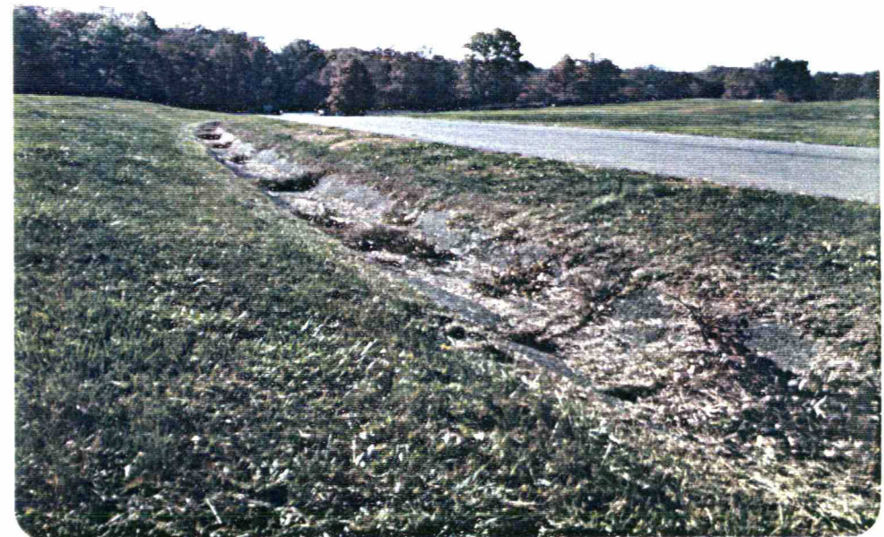
Ditch along Rte. 10 in Need of Cleaning
