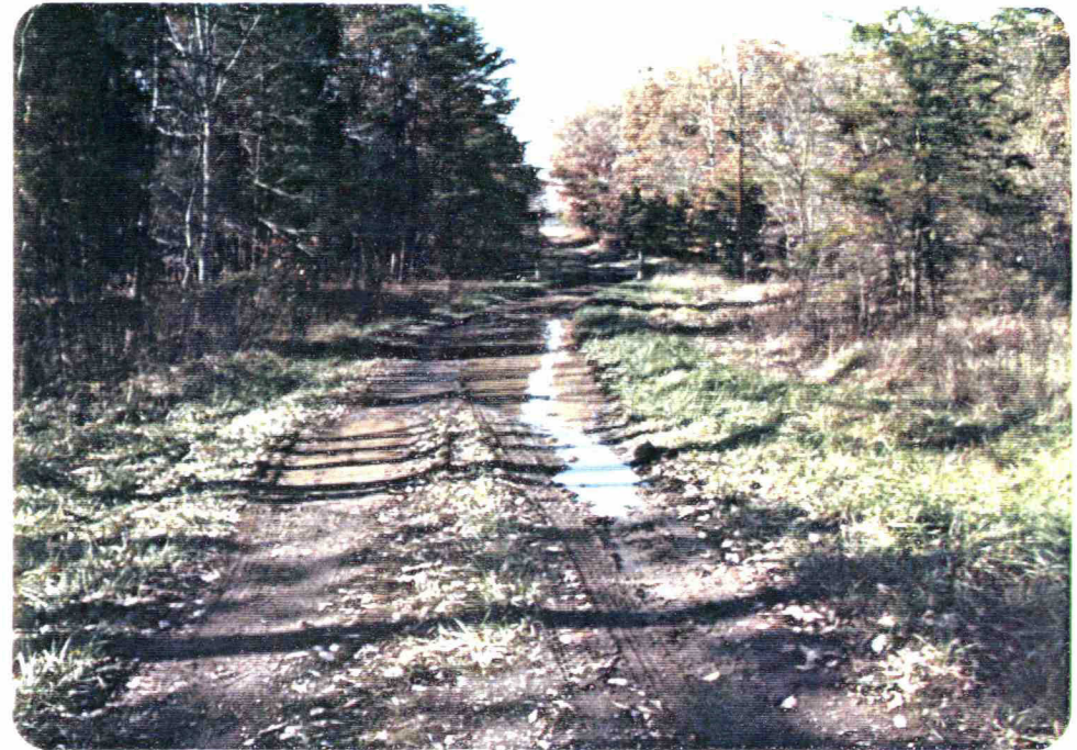
Poor Drainage on Rte. 410 at MP 0.12
