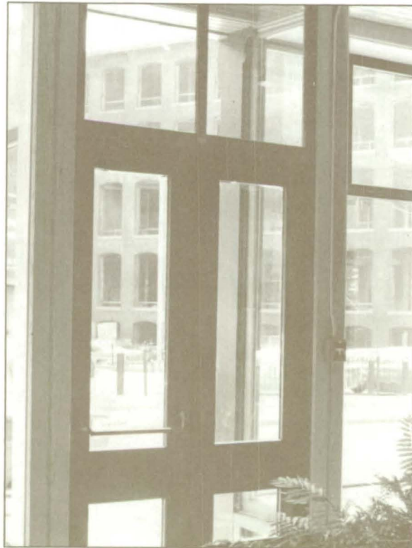
The building code requires two means of egress. This can often be provided in a way that preserves the character of original doorways.
