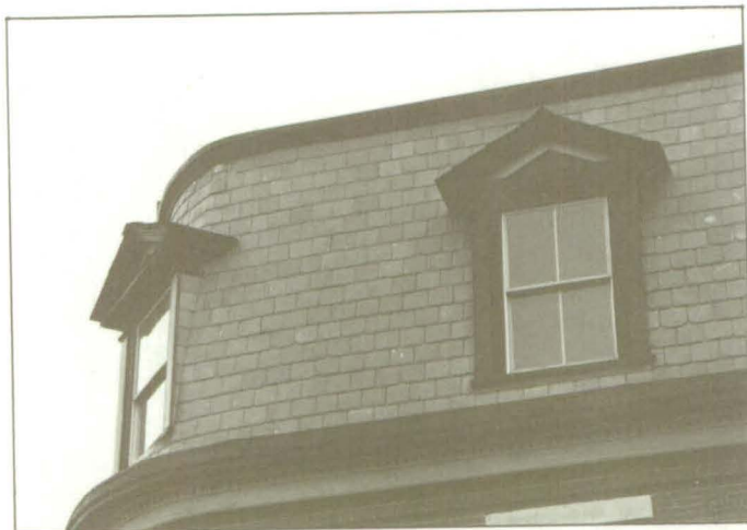
The shape of and materials covering roofs of historic buildings are important. Many of the remaining slate roofs in Lowell are in good condition and should be retained.
