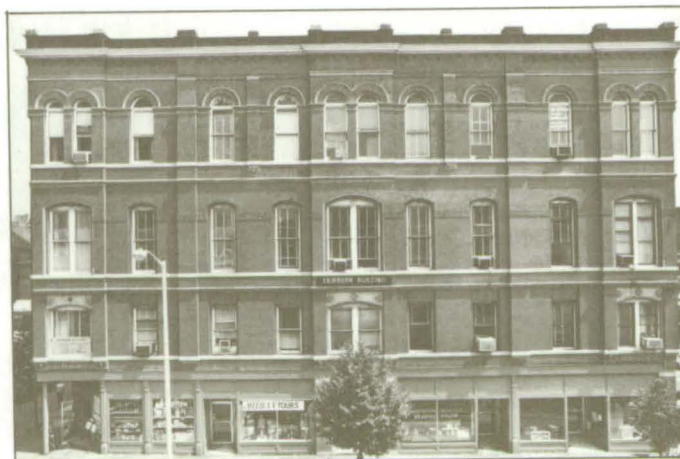
The recent storefront rehabilitation has revealed formerly covered historic materials and details. The building now exhibits an integrated 19th century appearance.
