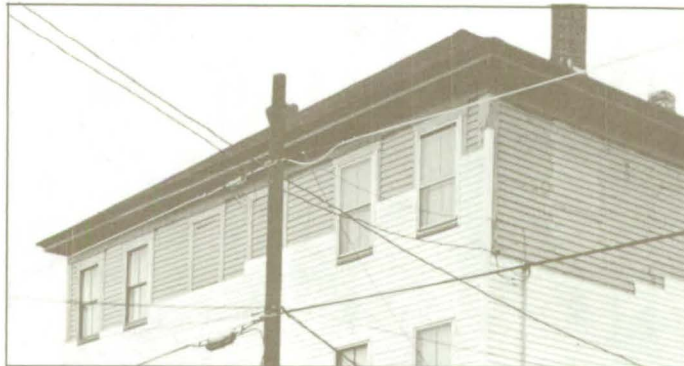
The application of synthetic siding can cause immediate or future damage to historic materials. The original window casings are being covered by vinyl siding.
