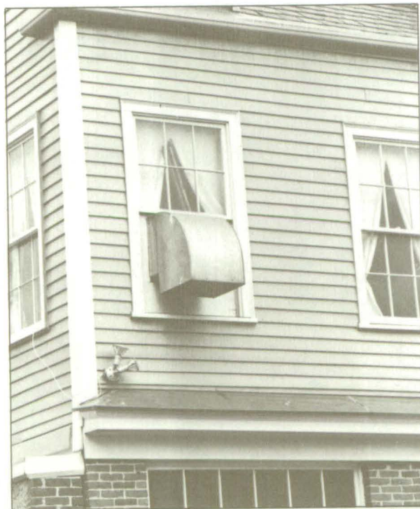
Intake and exhaust ducts and grilles are often necessary. Effort should be made to locate such features so that they do not detract, as in this case, from an historic facade.
