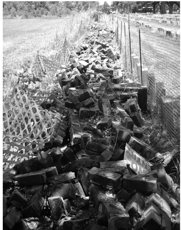
Figure 13-1. Damaged cemetery walls at Chalmette, 2008. (author)
