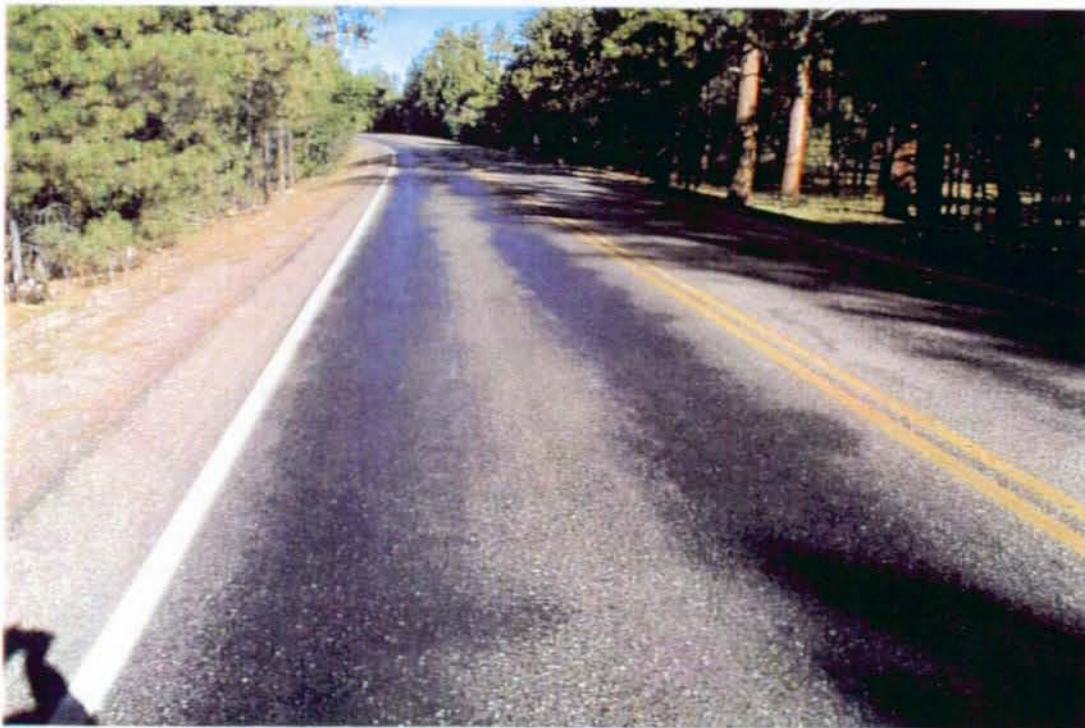
Photo #3709 - MP 8.44 - Heavy Bleeding, looking backwards.
