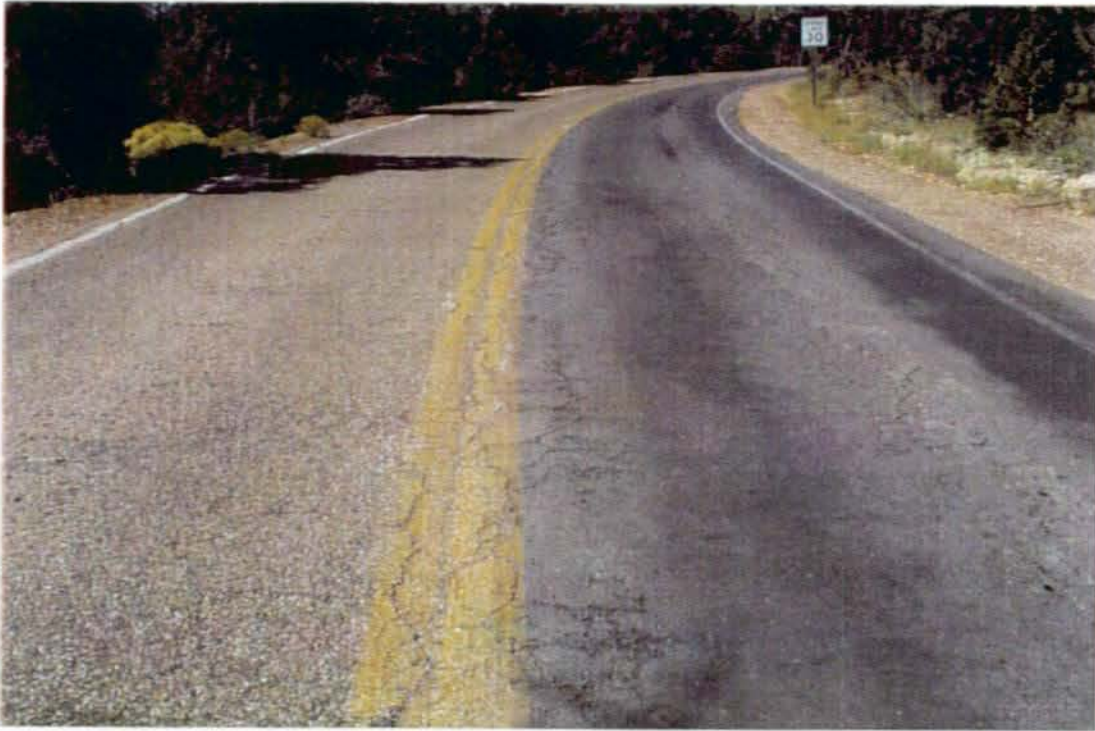
Photo #3684 - MP 0.50 - Asphalt in Westbound Lane, Old Chipseal in Eastbound Lane.
