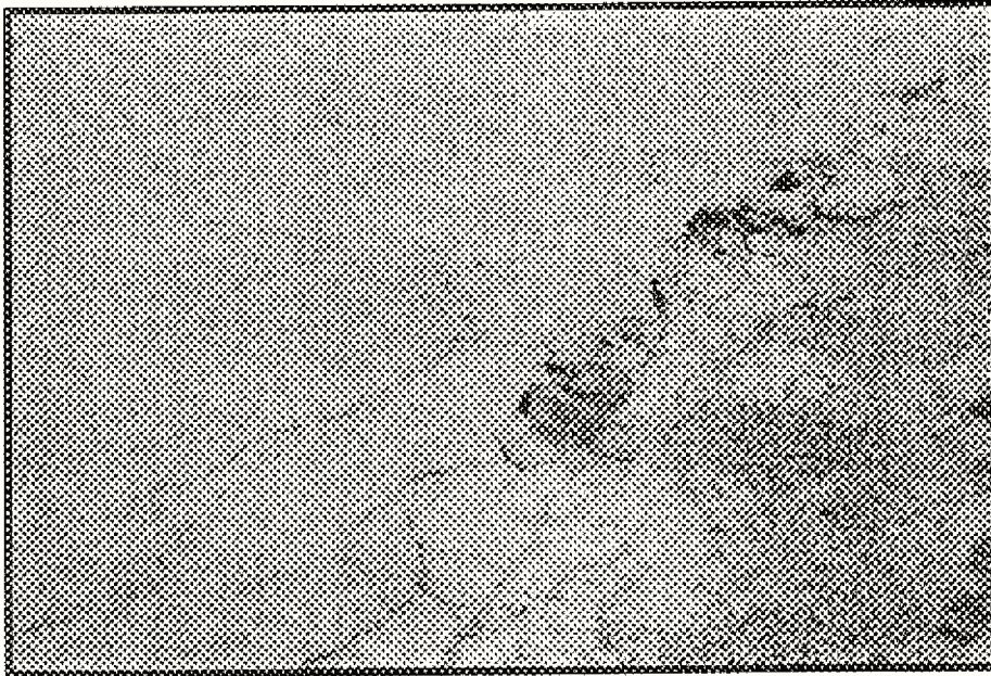
Photo # 33 - MP 0.24 Cobblestones protruding through pavement
