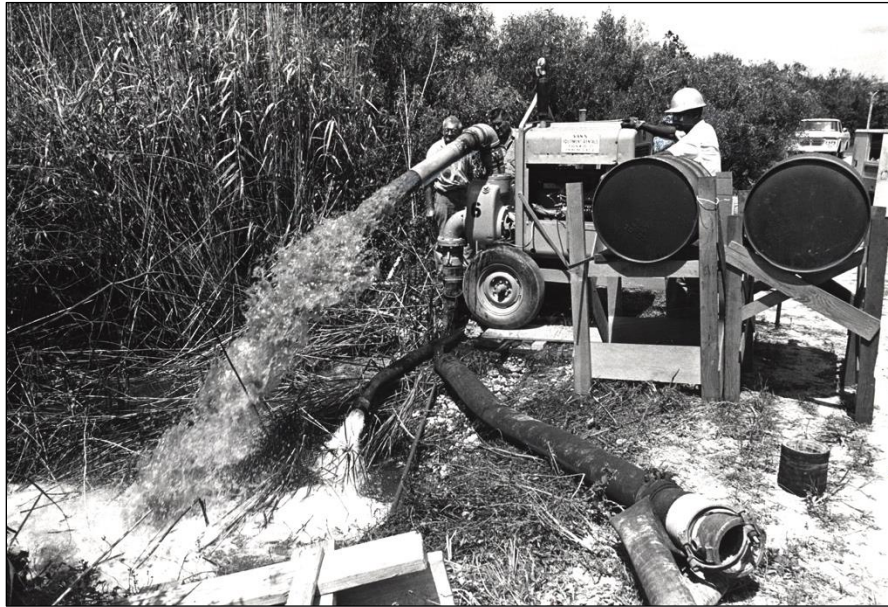
Figure 8-5, pumping from a well at the Anhinga Trail
