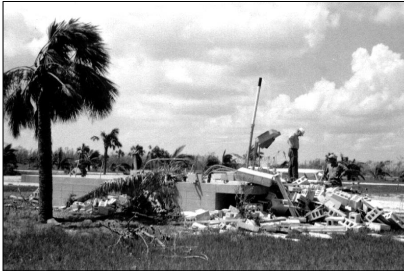
Figure 7-11, Flamingo comfort station after Hurricane Donna, Oct. 1960).
