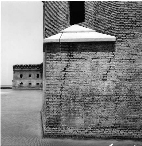
Figure 167. Vertical cracks at Bastion 1, 1970. (Alexander Physical Status Report 15)
