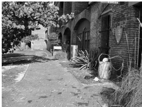
Figure 253. AC compressor on tour route, 2010. (SERO image 1493)
