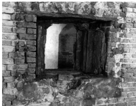
Figure 94. Typical lower tier embrasure showing exfoliation, 1970. (Alexander Physical Status Report 20)
