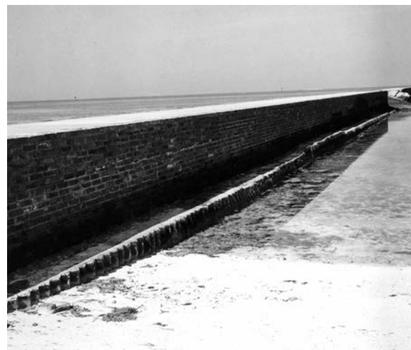
Figure 105. Counterscarp wall repair opposite Front 4 showing section in back washed out by Hurricane Betsy, 1970. (Alexander Physical Status Report 7)
