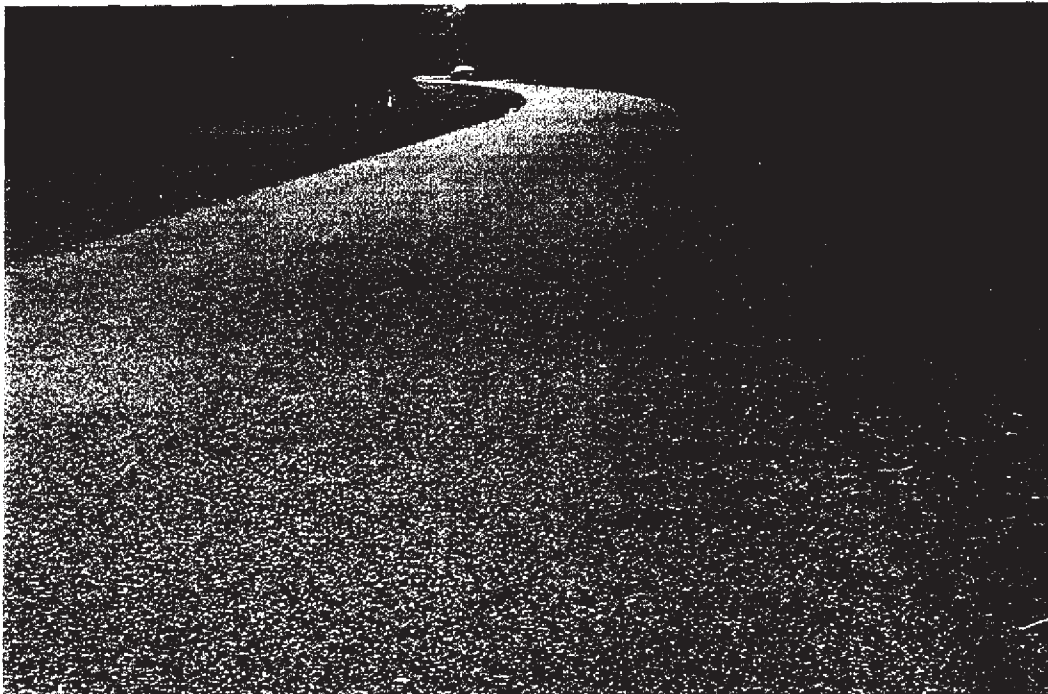
Photo #2915 - MP 0.60 - Localized pavement distress
