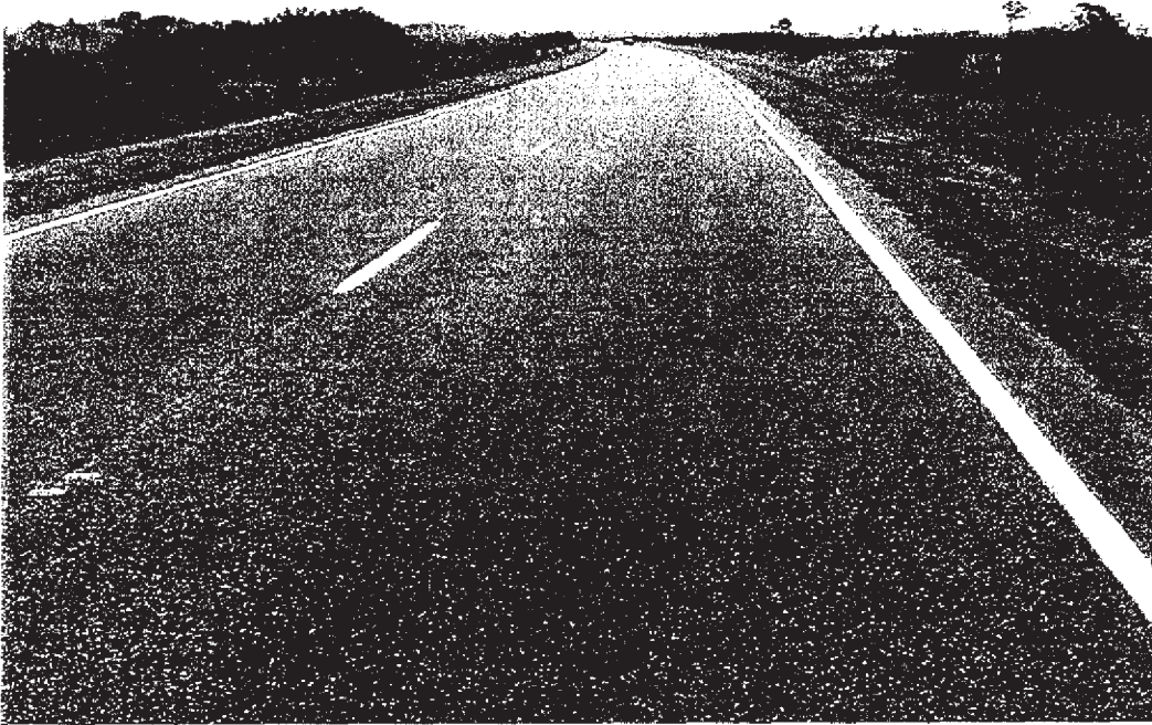
Photo #2911 - MP 3.30 - Typical pavement section with corrugations
