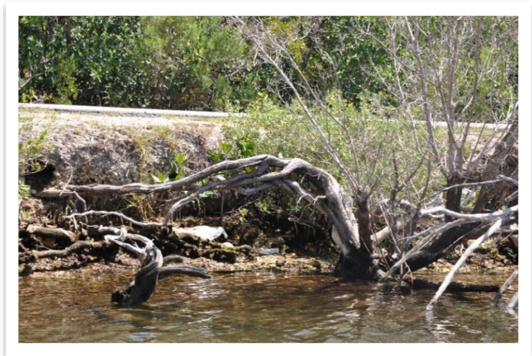
Figure 2. Erosion along the Convoy Point Entrance Road at BISC, May 2015. PSDS photo.
