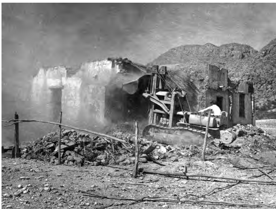
Figure 6–III.142 NPS employee razing the Chata Sada house at Boquillas in the 1950s.
