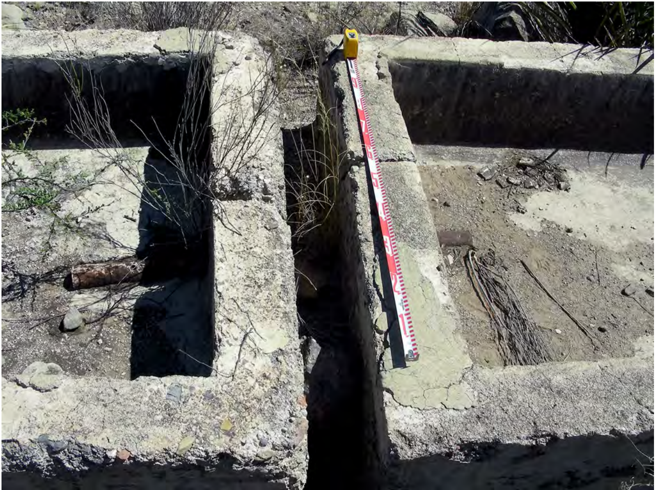
Figure 6-III.31 Concrete water troughs connected in series at BIBE991 (41BS2286). Photo by D. Petrey.
